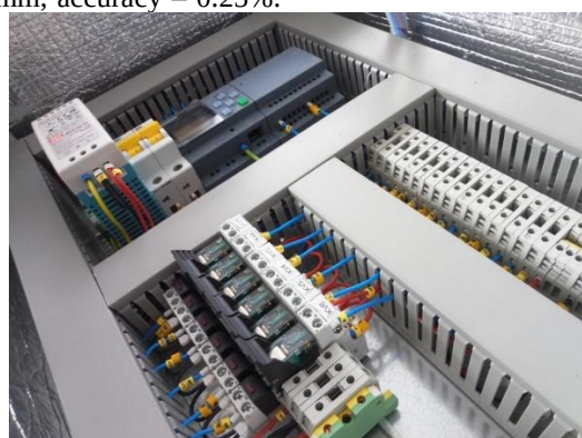
Fig. 4. The control cabinet of the hydraulic drive for the synchronous motion of working bodies in machines
